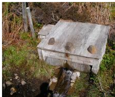
A 500W hydro for battery charging showing tailrace
