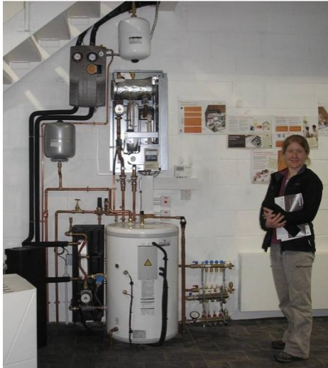
The Daikin Altherma Air Source Heat Pump, Active Energy, Inverness
